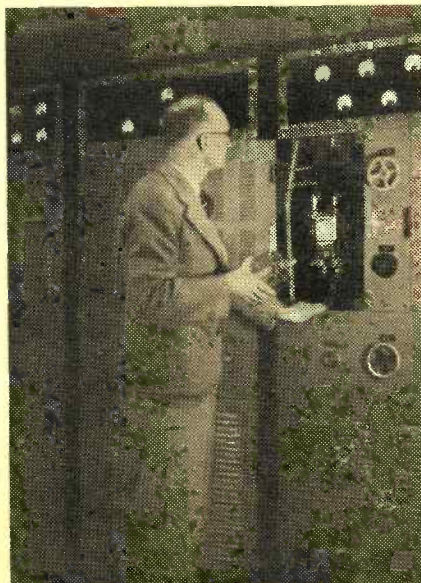
● Chief Technician Bert Sctrine (VK3BI) holding one of the 833 Class B modulators at the transmitter.
